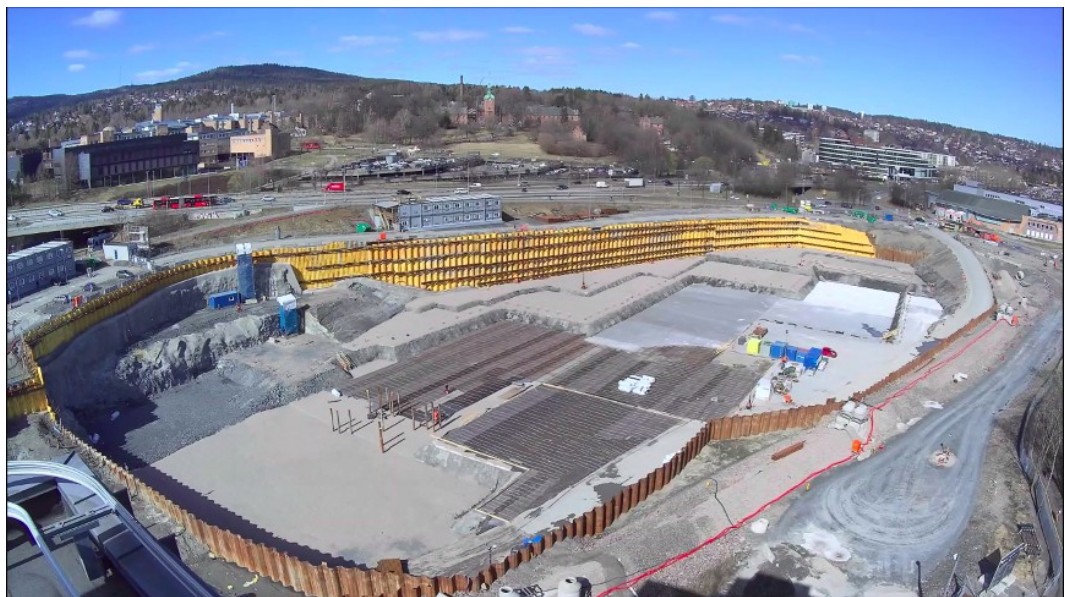
Figure 7: Image of the construction site of the LSP. Retrieved from organizational document, see table 1.
