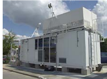
Source: Norsk Hydro - Norsk Hydro Electrolysers supplied the hydrogen producing electrolyser technology at the Hamburg fuelling station
