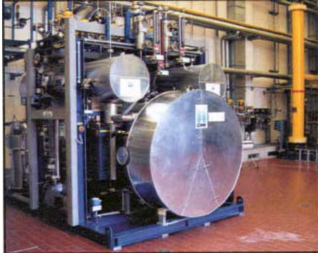
The interior of the GHW electrolyser
