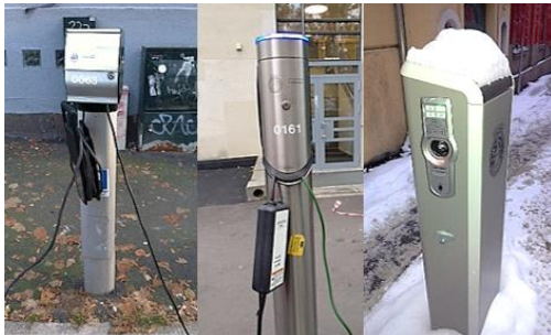
Picture 5: Three generations of charging stations in Oslo
