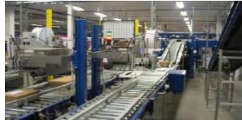
Picture 26: Conveyor belts
